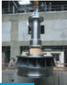
San Roque, 3 × 137MW Water-Turbine/Generator
