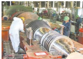
Central power generation station at Tokuyama Corporation's Tokuyama Plant
