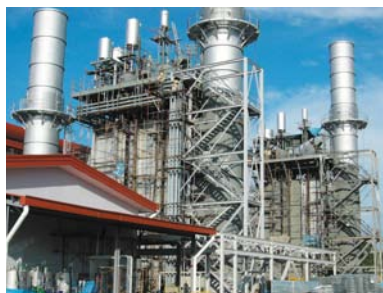
Combined cycle power plant (Dar Es-Salaam, Brunei)
