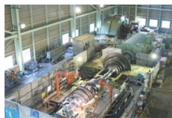
No. 2 power plant at Tosoh Corporation's Nanyo Complex
