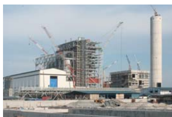
Jimah coal-fueled thermal power plant (Malaysia)
