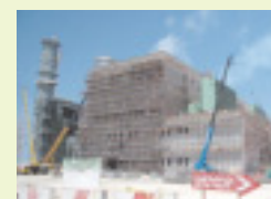
Sidi Krir power plant
