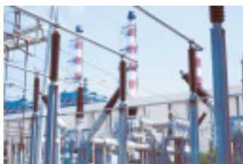
Muara Karang switching station and substation (Indonesia)
