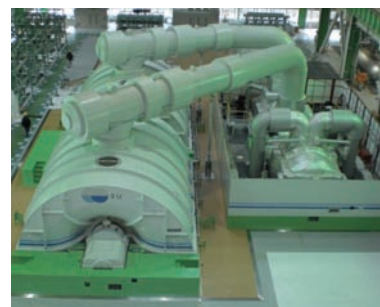
Maizuru Power Station, The Kansai Electric Power Co., Ltd.
