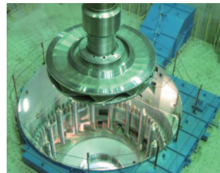
Kannagawa Hyrdoelectric power plant, The Tokyo Electric Power Company, Inc.
