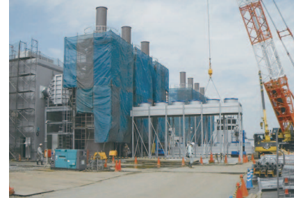
Nihon Techno's Sodegaura Green Power Project
