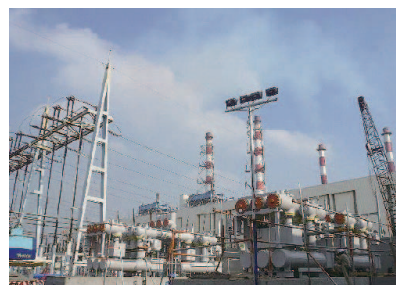
Muara Karang Substation
