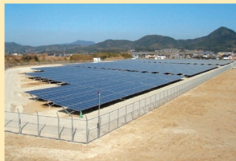
Mega-Solar Tsuyazaki No. 1 Power Station, MM Energy Co., Ltd.
