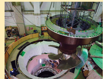
Generator unit 5 at the Tohoku Electric Power Miyashita Power Plant (39 MW)
