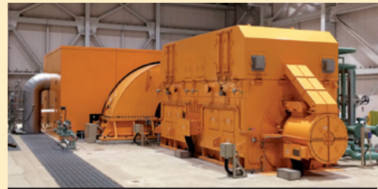
Steam turbine generator (Saiki Power Plant, erex New Energy Saiki Co., Ltd.)
