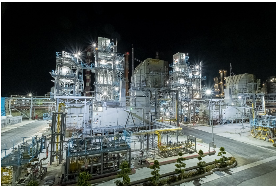
CHIMEI Corporation Gas Turbine Cogeneration System 2 x 30MW
